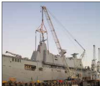
▼ An SyncHoist system used to align steel blocks of the ship's control tower sections allowing gradual lift and positioning of the load.
