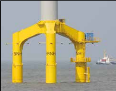
▲ Offshore wind turbines levelling: Enerpac's synchronous lifting system provided the solution for levelling the supporting cross pieces for 80 wind turbines.
